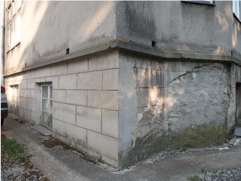
Figure 6-7: Signs of frost damage in the plinth area of a building that has log walls with ventilation cladding and plastered finish. On the right-hand side, the old plaster has delaminated from the limestone masonry. On the left-hand side, the plinth has been renovated, but early signs of deterioration are already visible in the lower section. Photo: Paul Klöšeiko.
