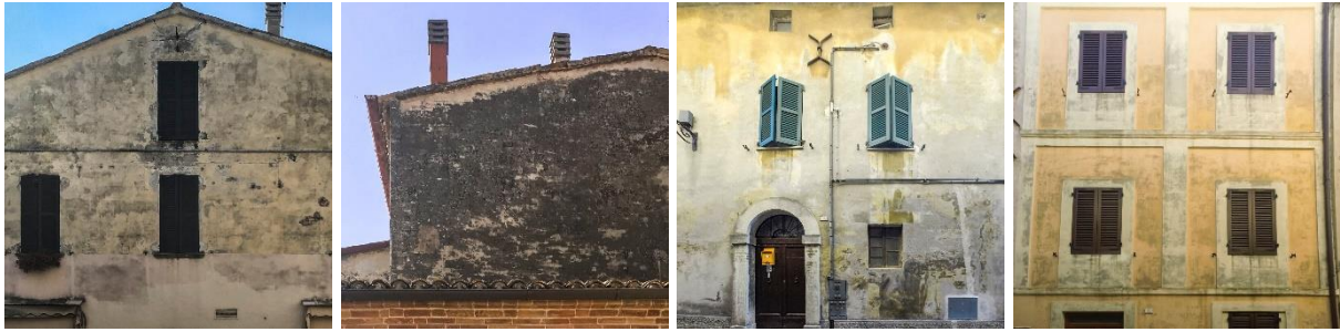
Figure 3-7: Examples of algae growth on external walls: (left two) façades exposed to wind driven rain; (right two) fed by drain water from windows overhangs (Blumberga and de Place Hansen, 2020 and https://www.ribuild.eu/algae-growth )
