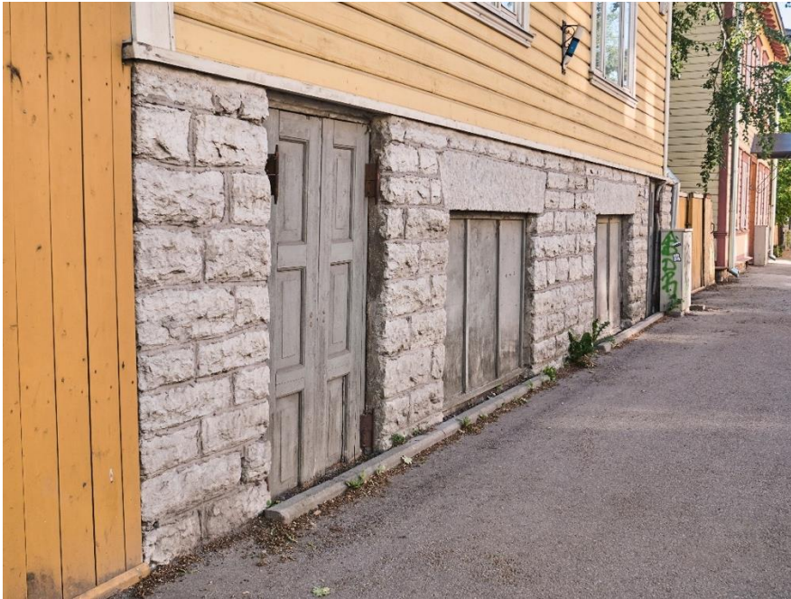
Figure 6-6: Limestone plinth area that has been submerged below the asphalt surface. An additional barrier made from kerbstones to prevent street surface runoff from entering the windows has proven to be insufficient. Photo: Paul Klõšeiko.
