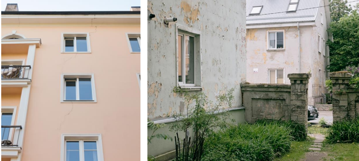
Figure 6-8: Cracks in the plastered mass masonry wall that have reappeared after replastering (left). Too vapour tight paint has started to peel off (right). Photos: Paul Klõšeiko.
