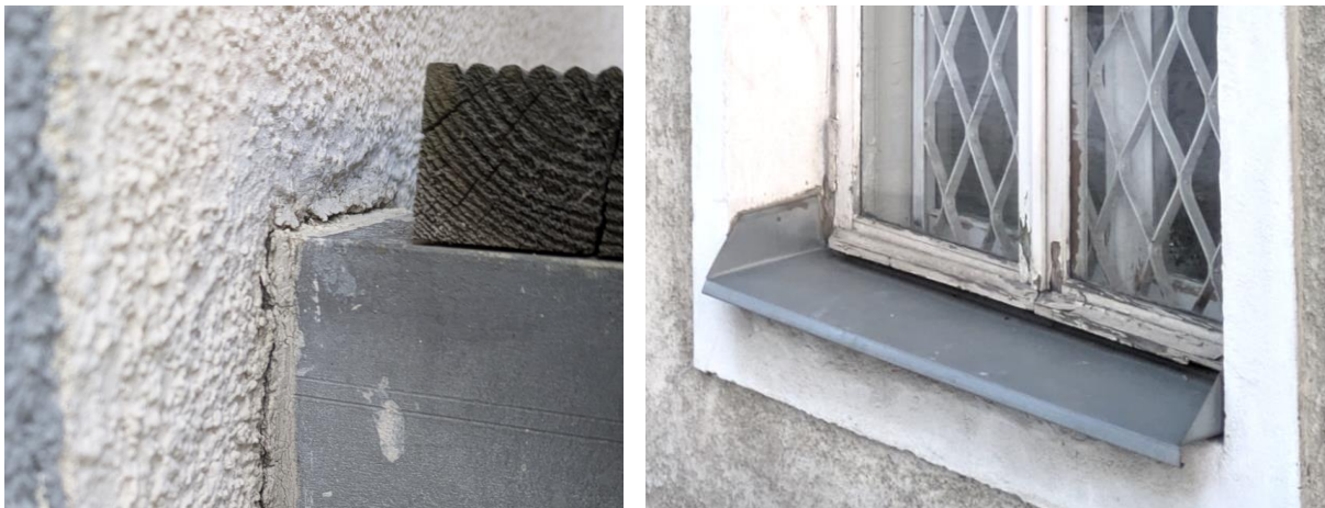
Figure 3-6: Sealant is damaged by UV radiation and differential deformations (left). Shrinkage and swelling of the wooden window frame has contributed to degradation of the paint layer (right).
