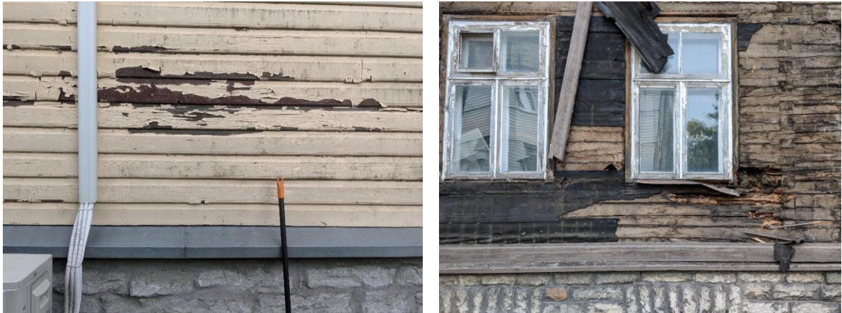
Figure 6-5: Condition of painted wooden cladding (left); damage to the load bearing structure due to faulty window flashing becomes visible after removal of the cladding (right). Photos: Paul Klõšeiko.
