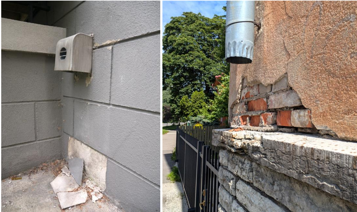
Figure 6-9: Left: lower section of the ETICS plinth, where plaster is in direct contact with the concrete strip cast against the plinth surface. Right: damage is commonly tied to faulty rainwater systems highlighting the importance of timely maintenance. Photos: Paul Klöšeko.
