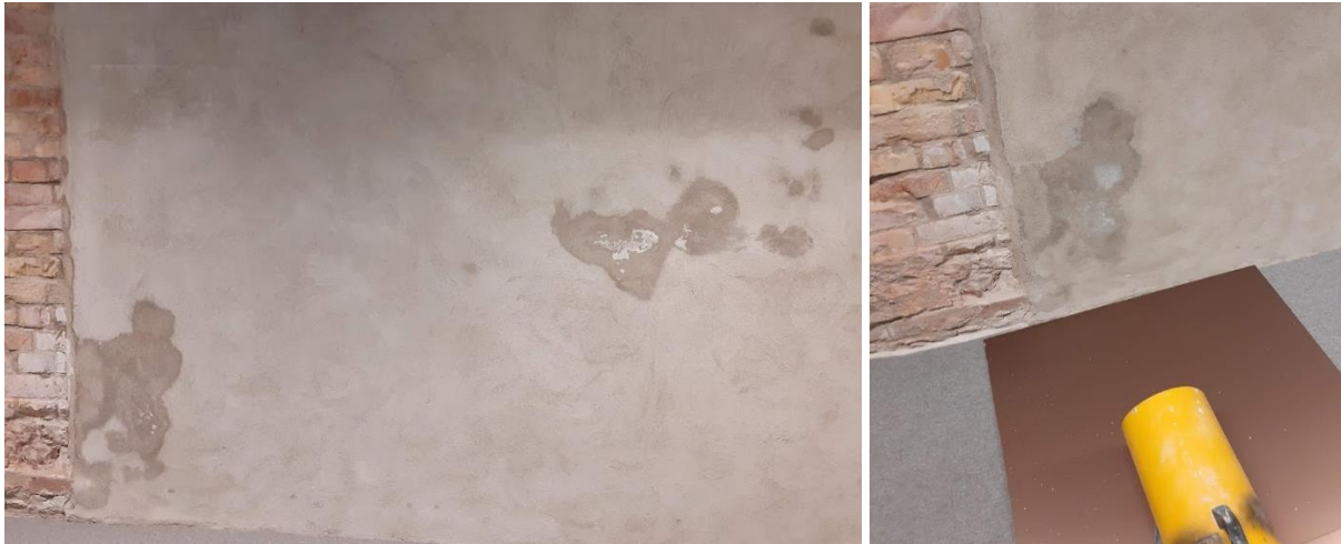
Figure 3-2: salt efflorescence appearing on damp areas of a masonry wall finished with cement-lime plaster after renovation (left). The moisture source was precipitation that infiltrated the masonry cavities during the renovation process. Drying was accelerated using localised heating to halt further salt migration (right). Photos by Martin Talvik.
