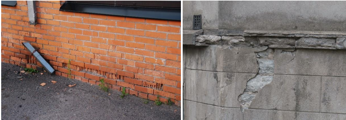
Figure 3-1: Left: frost damage in the plinth area of a brick wall. The bricks lack adequate frost resistance, making them unsuitable for use in plinth areas exposed to freeze-thaw cycles in cold climates (photo: Targo Kalamees). Right: damaged water flashing on top of plinth has led to frost damage of underlying lime-sand bricks and plaster below (photo: Paul Klõšeiko).
