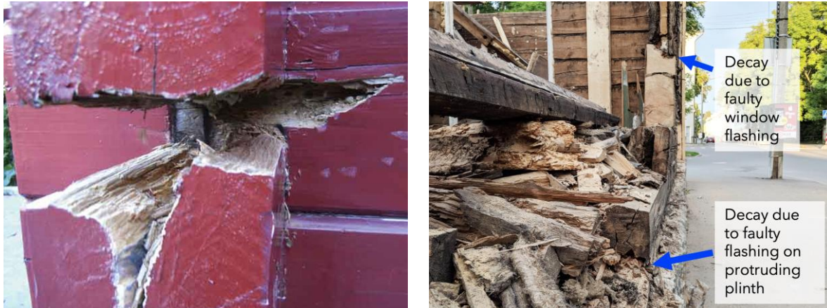
Figure 3-4: Left: rot damage at the notch joints in a log wall (photo: Sverre Holøs, SINTEF 720.082, 2007). Right: rot damage of logs behind ventilated cladding, caused by faulty flashings (photo: Paul Klößeiko).
